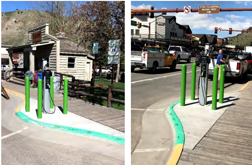
FIGURE 6.5: ON-STREET EV CHARGING STATION
