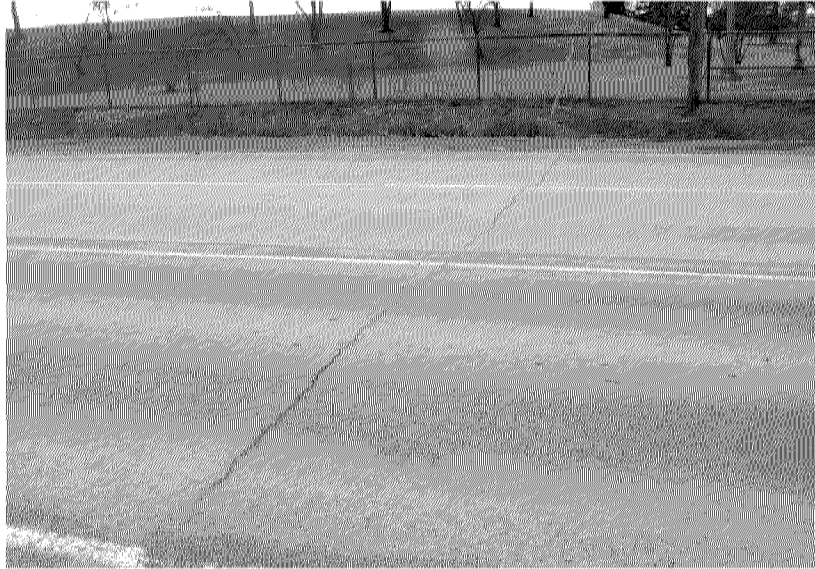
Transverse /Thermal cracking
