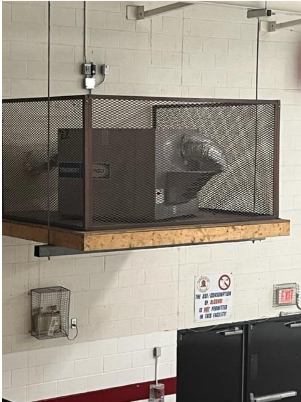
SCRC Pad 1 dehumidifier replacement
